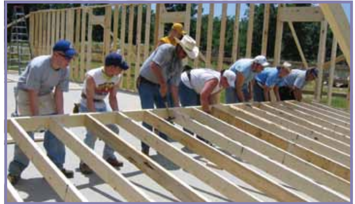
Student participants in the 2004 Ringold, Oklahoma, mission help with the framing of a building.
